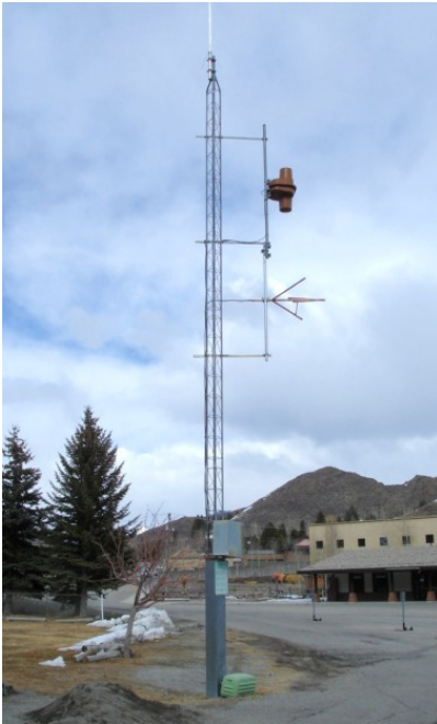
Tower with two co-located low power antennas connected to transmitters in building closet via 140ft underground conduit
