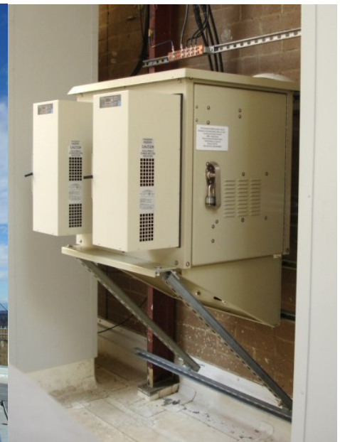
Equipment cabinet containing transmission equipment for antenna pictured left
