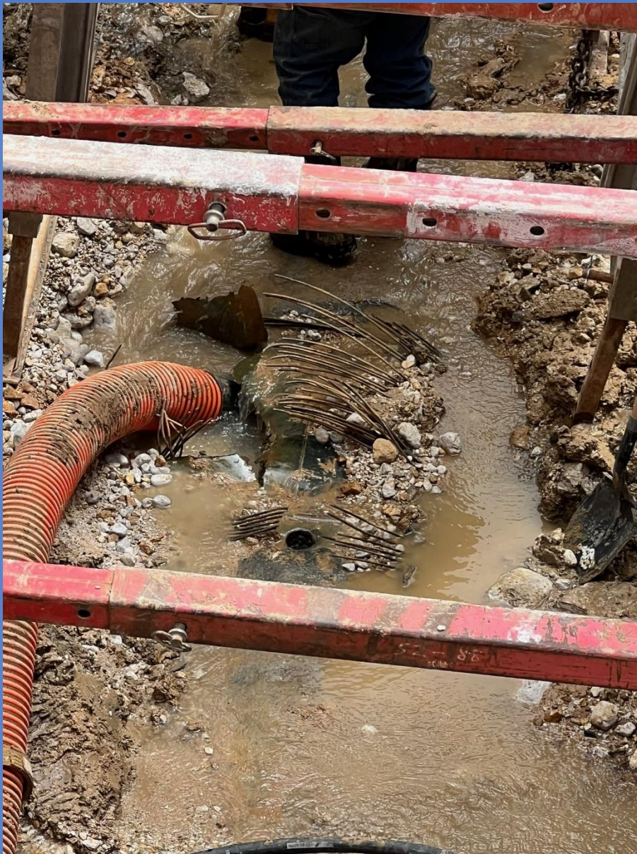
Top of failed pipe
