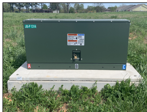
THREE-PHASE PRIMARY JUNCTION BOX
