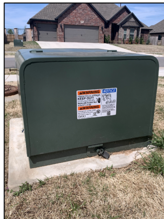
SINGLE-PHASE PADMOUNT TRANSFORMER
