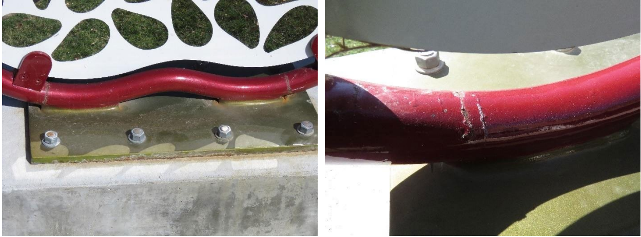
(Left) The green self-base, which shows loss of finishes on the sides, with corrosion of exposed metal. There is also white hazing from calcium deposits. (Right) Loss of finishes and corrosion of the metal on the red “peel” of the apple are most apparent at seams.
