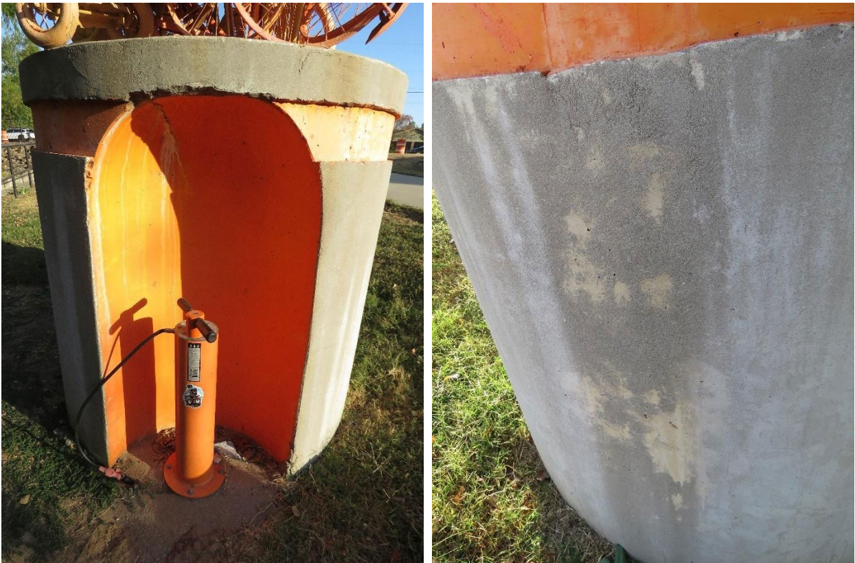
(Left) A crack at the top of the niche, with fading of the paint finishes. (Right) Irregular cementitious parging on the concrete base.
