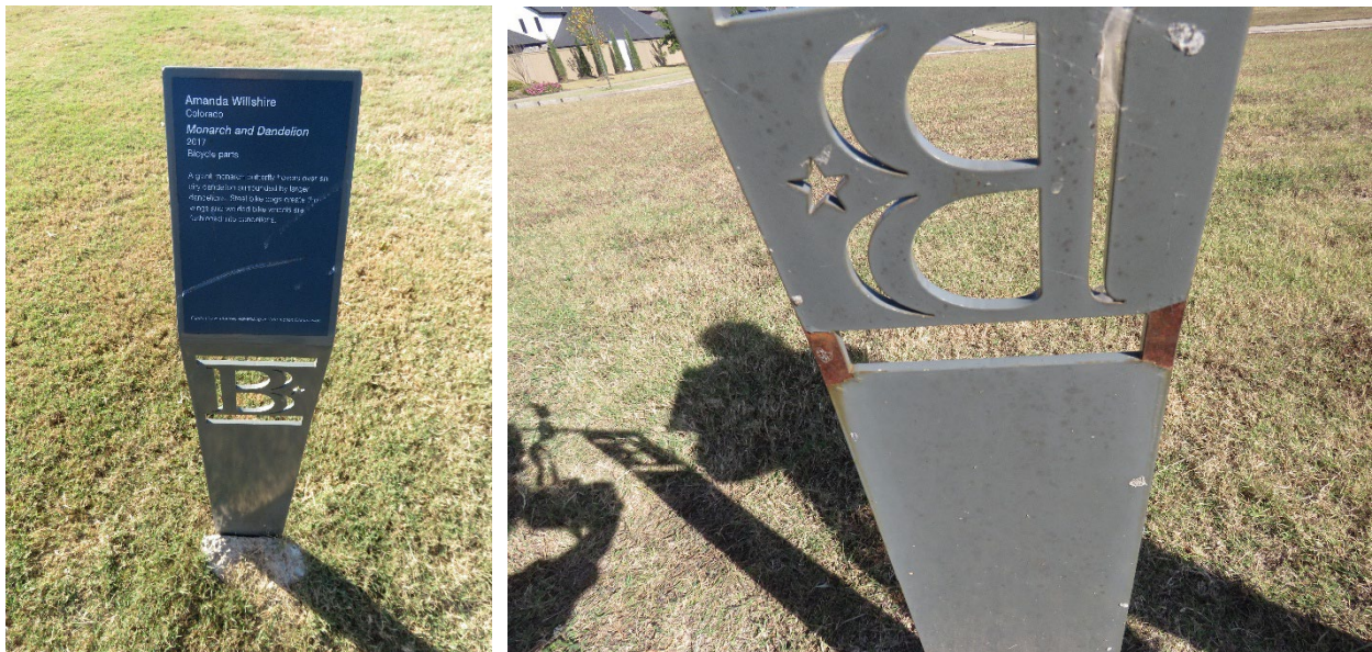
(Left) Abrasions on the label for Monarch and Dandelions. (Right) Loss of paint finish and corrosion of exposed metal on the back side of the sign for Open Heart.
