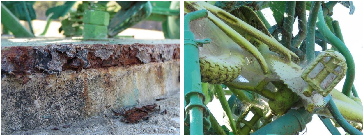
(Left) Heavy corrosion on the side of the metal self-base. (Right) There is a significant amount of insect nesting.
