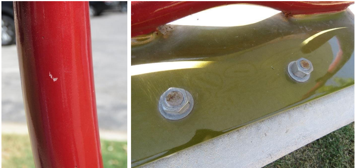
(Left) Small abrasion, with loss of the finish, exposing the primer. (Right) Mild corrosion of the hardware.
