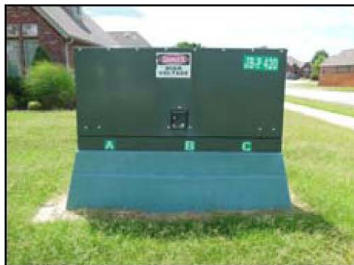
SINGLE AND THREE PHASE JUNCTION BOXES
