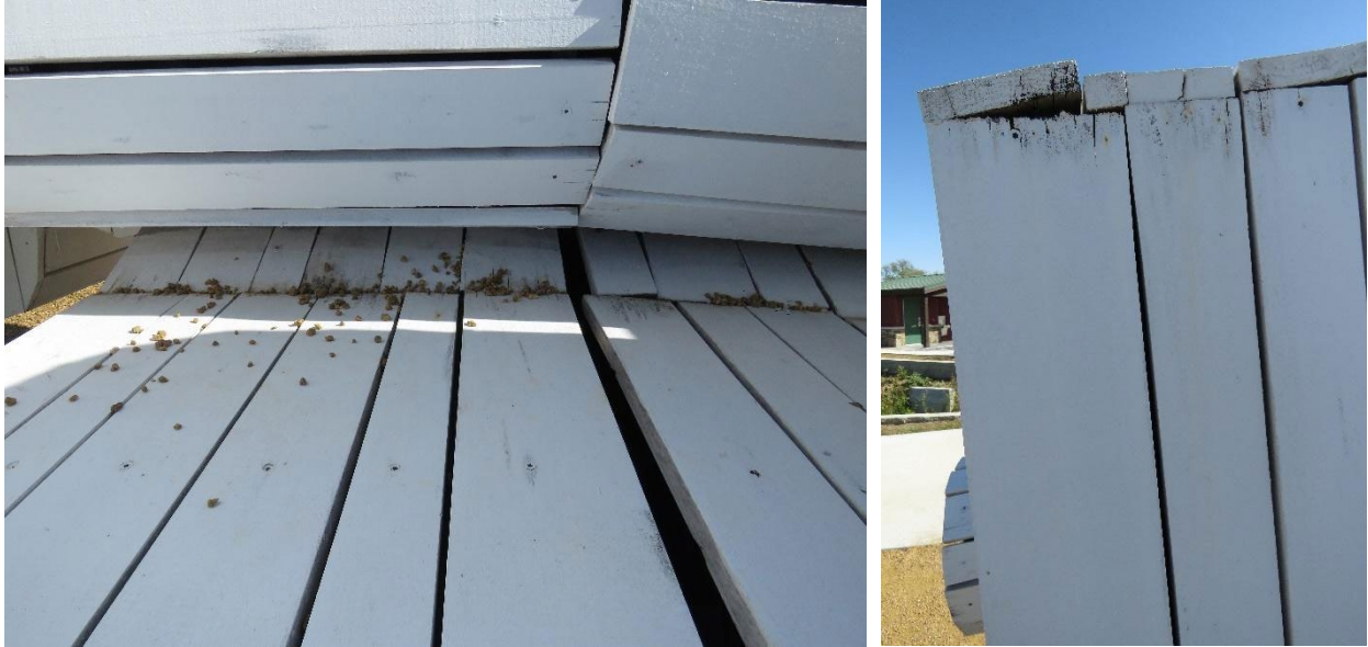
(Left) Bits of gravel observed on top of the sculpture. (Right) A board that is slightly detached and lifting. Note the minor splits at the edges of the boards.
