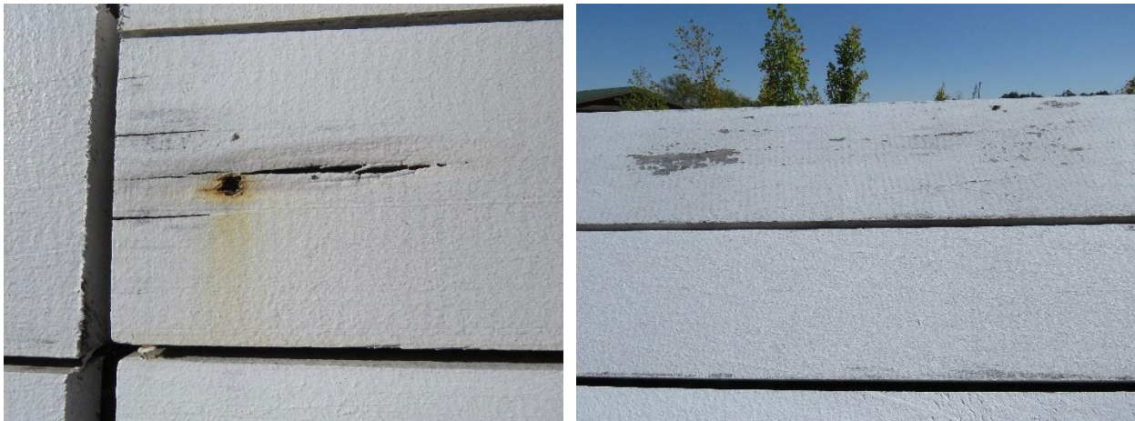
(Left) Corrosion of the hardware and associated iron staining on the painted surface. (Right) The paint has been thinly applied in areas, with losses and flaking observed.
