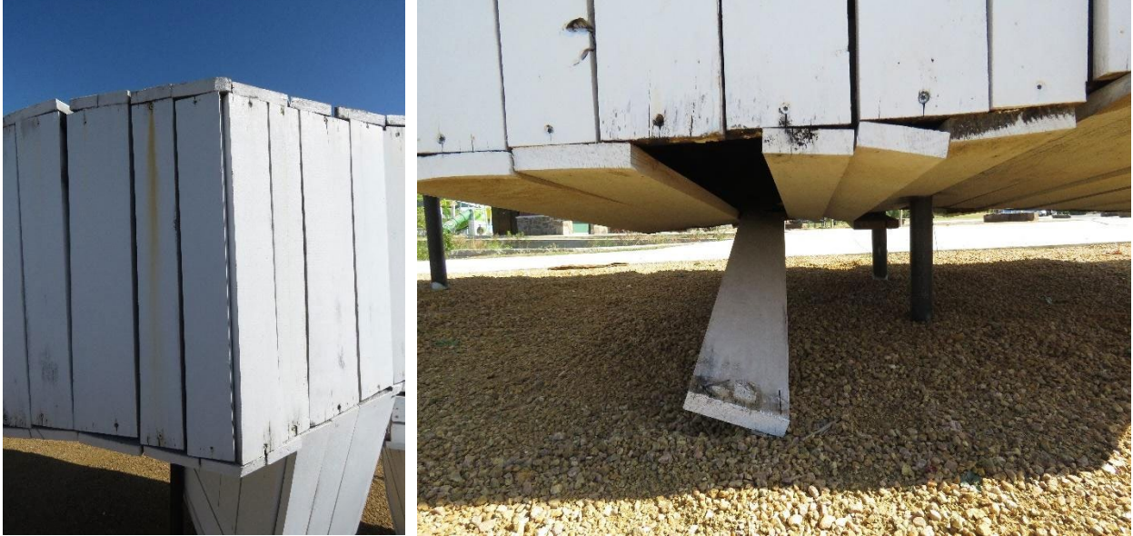
(Left) Displacement of boards and iron staining from corrosion of hardware. (Right) A detached board on the underside, held in place at one end.
