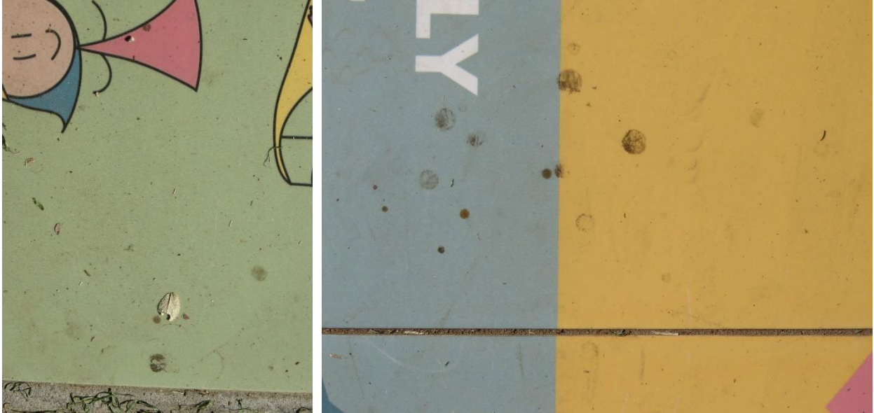
(Left) Soiling and debris on surfaces. (Right) Biological accretions and scuff marks.
