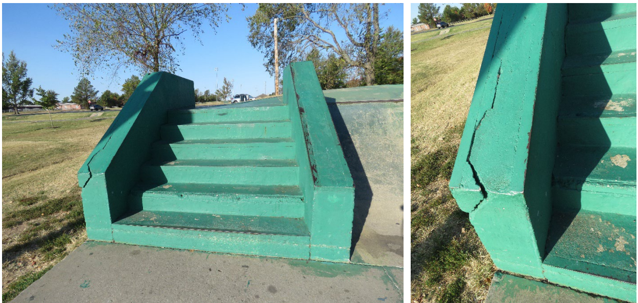
(Left) The stairs located south of the bowl, on the western end of the skate park. (Right) The south concrete bannister exhibits pronounced cracking at top. Note also losses in the paint finishes on the stair treads.
