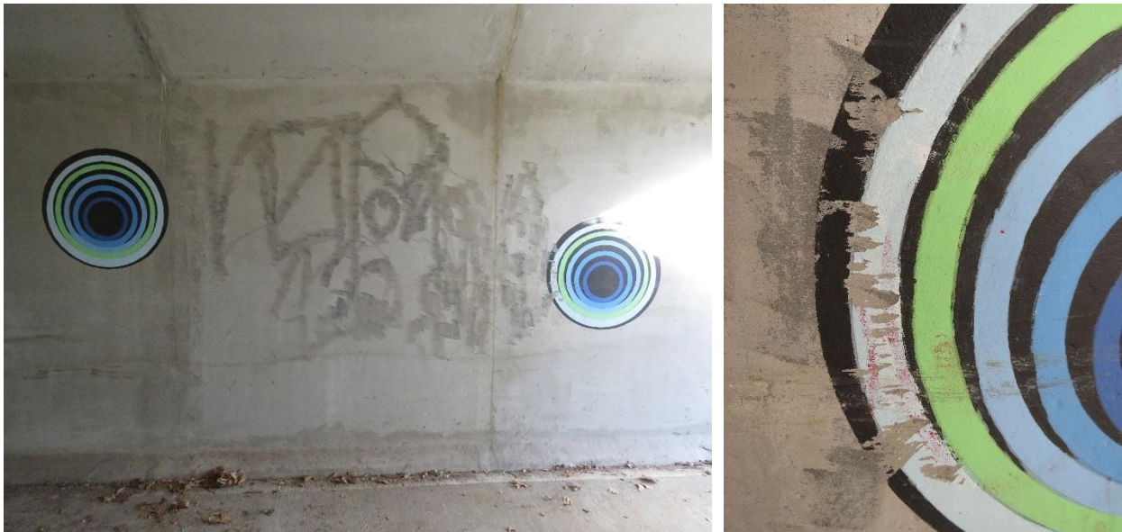
(Left) Large area of graffiti between circles on the east wall. (Right) Abrasions and paint loss, with red crayon graffiti markings.
