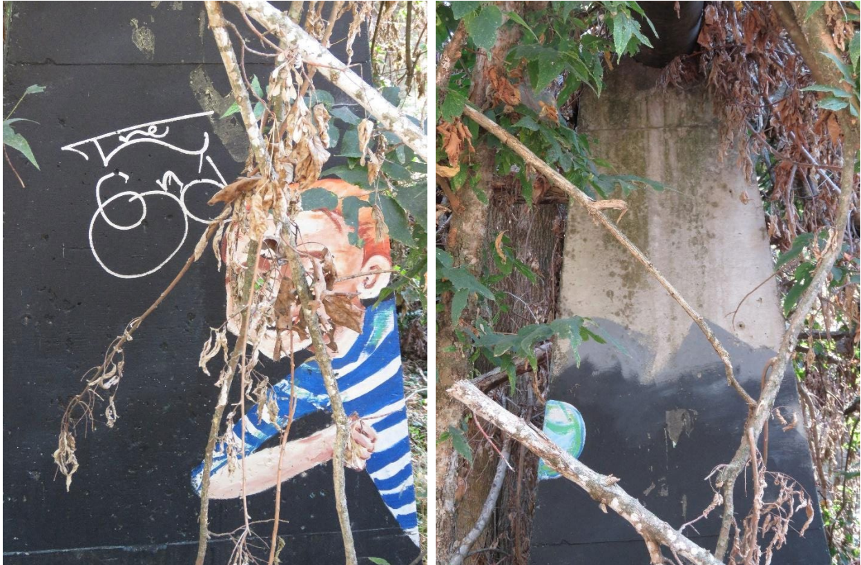
(Left) Similar to the first pillar, the second pillar is more easily accessible to the public and contains graffiti markings. (Right) Pillar two has heavy biological growth around the top.
