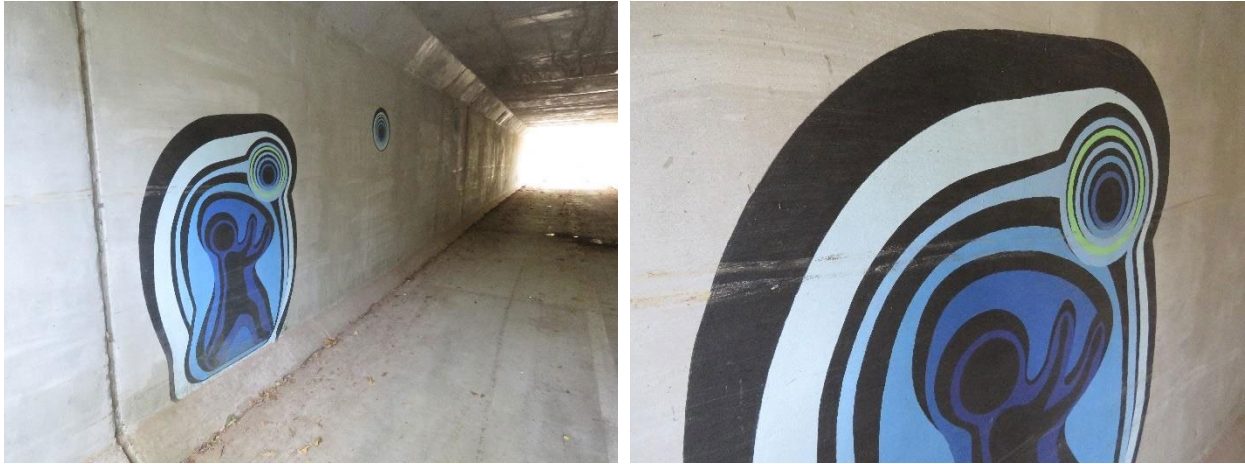
(Left) The east side of the tunnel, with the basketball player next to the north entrance. (Right) Linear abrasions observed on the mural.
