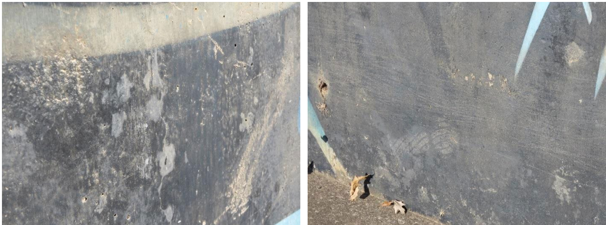
(Left) Cracking in the concrete and bubbling and peeling of the anti-graffiti coating. Note also the heavy soiling. (Right) Linear abrasions on the mural, in an area outside the tunnel.
