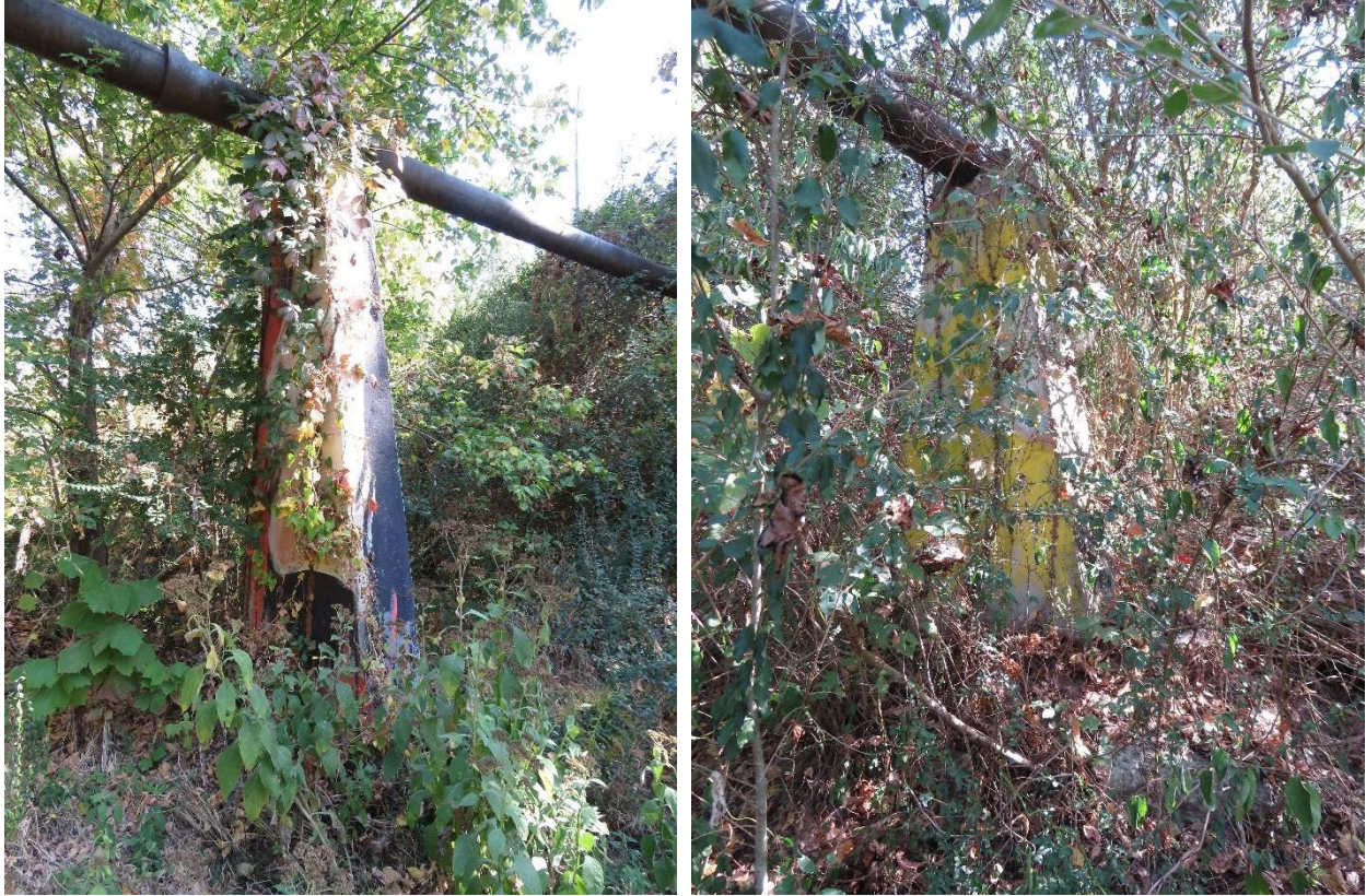
(Left) One side of pillar four has heavy plant encroachment and vine attachment. (Right) The easternmost pillar, or pillar five, is completely engulfed in plants and cannot be easily accessed.
