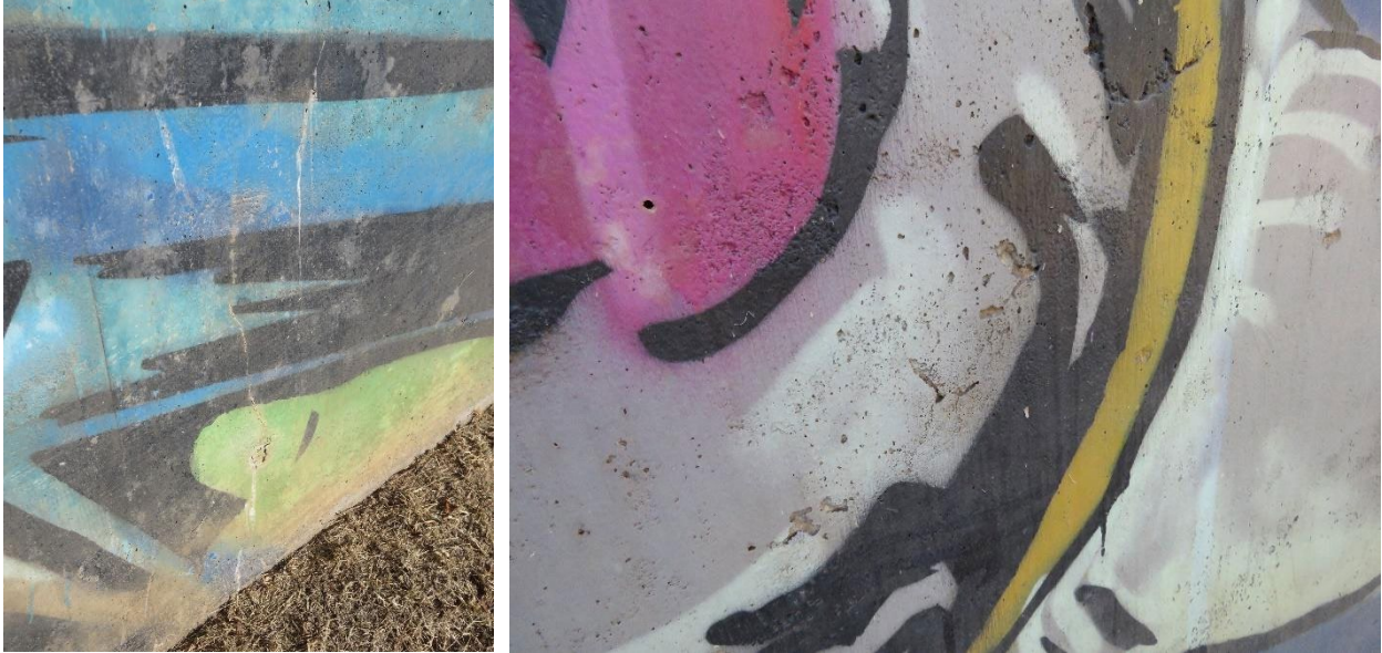
(Left) Cracking in the concrete with mineral deposits leaching out of the cracks. (Right) Voids and cavities in the concrete, small areas where paint did not reach.
