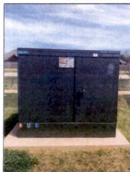
THREE-PHASE PADMOUNT TRANSFORMER
