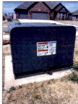
SINGLE-PHASE PADMOUNT TRANSFORMER
