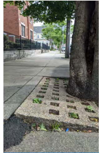
Tree Grate Conflicts
