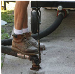
A technique for lifting concrete panels when they have sunk or collapsed.
