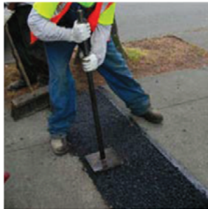
A temporary measure to smooth a cracked or lifted sidewalk, typically done with asphalt.
