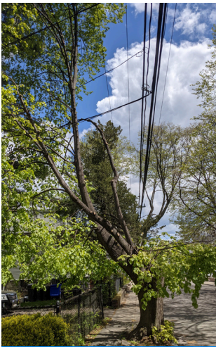
Overhead Utility Conflicts
