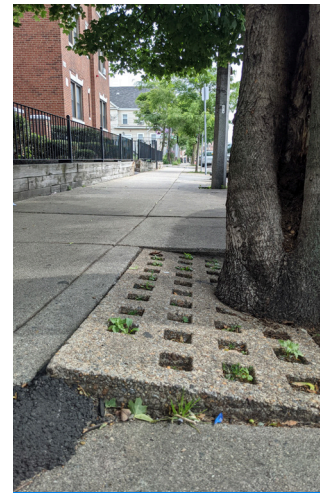
Tree Grate Conflicts
