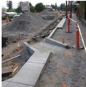
An open-graded gravel base course under the sidewalk to discourage root growth.
